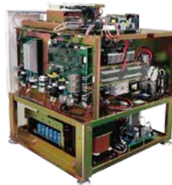
32kW / 40kW Super Capacitor Bank (PSU Generator)
